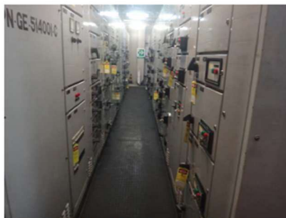
Painel Elétrico - PN-GE-514001C
