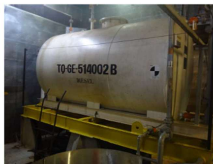
Tanque Diesel TQ-GE-514002B
